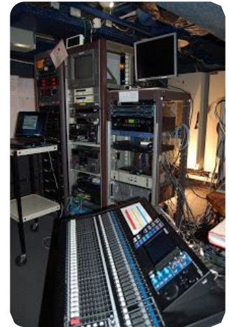
Cinema control room
